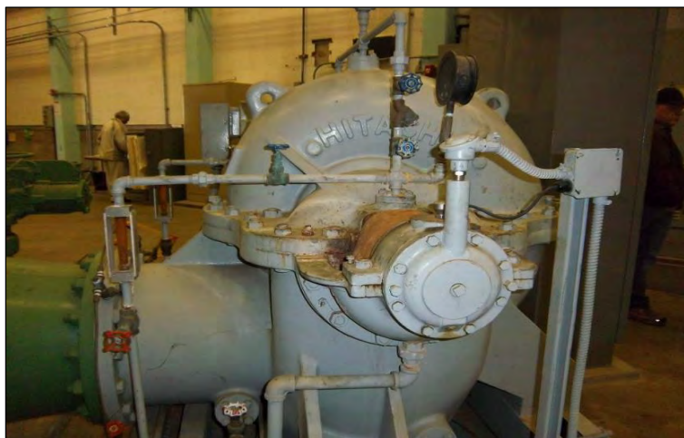
Vasona Pumping Plant pump
