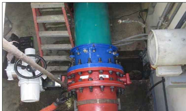
A typical rehabilitated line valve assembly
