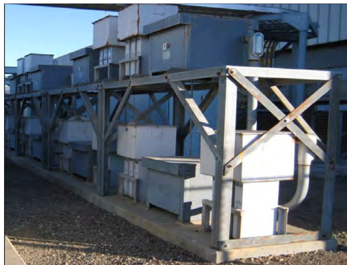
ASD motors at the Coyote Pumping Plant
