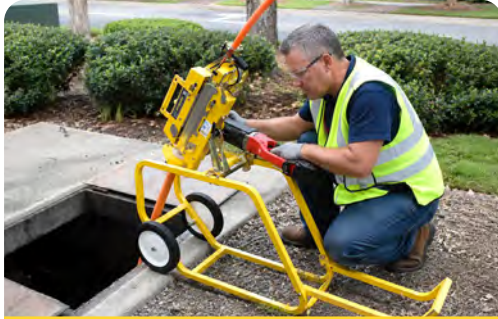
Outside Plant Fiber Optic Runs
