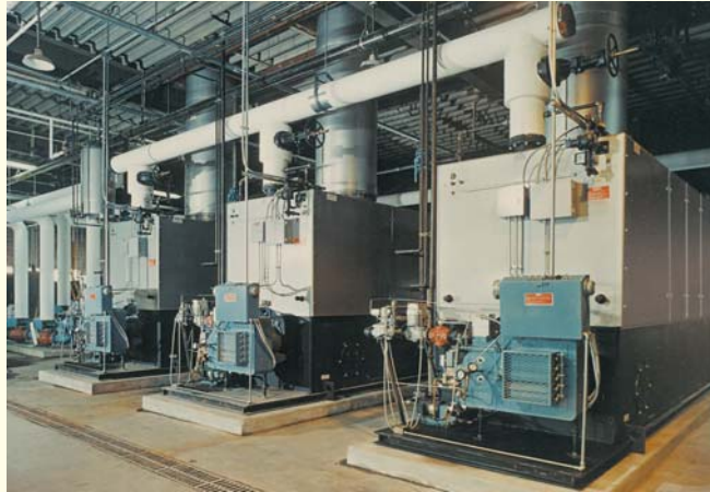
Three Bryan Boilers provide 56,250 MBH to heat 495,000 sq. ft. expansion of Milwaukee's General Mitchell Field air terminal.
