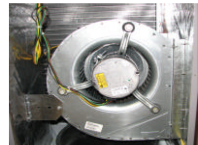
FIG. 2- Blower motor installed
