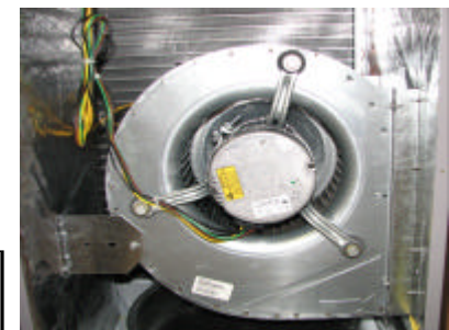
FIG. 2- Blower motor installed
