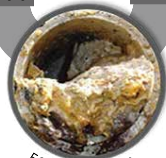
F.O.G. Blockage In Pipe
