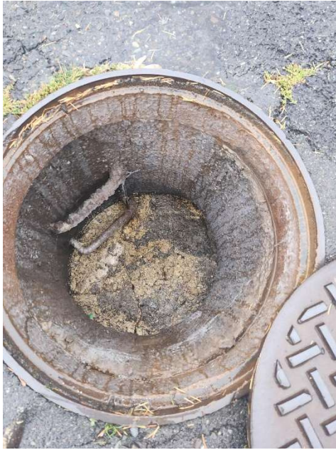
Sewer Plugged by Grease on Eatonville Hwy
