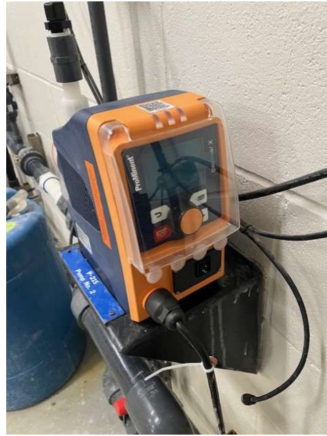
New Coagulant Pump Install Water Plant
