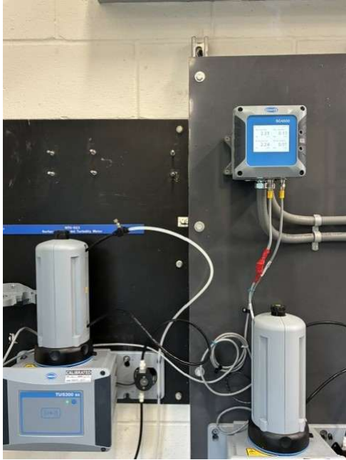
Surface water turbidity meter install completed
