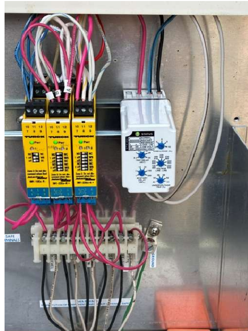
Phase Monitoring Installed on Sewer Lift Stations
