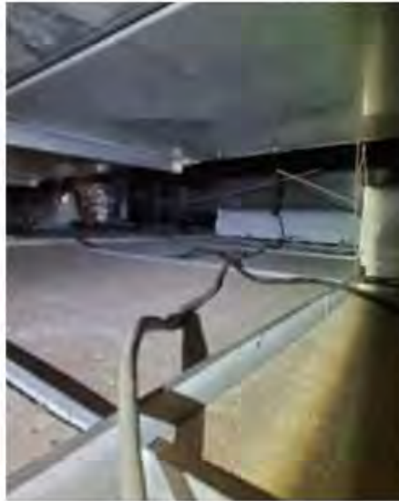
12) Spray-on fireproofing material scattered across the surface of drop-down ceiling tiles.
