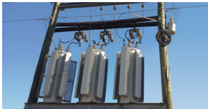
GE's Pole Mount Voltage Regulator (VR-PM) installed on a platform in a distribution network
