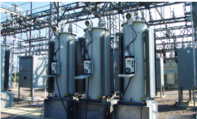
GE's Substation Voltage Regulator (VR-SS) installed on a distribution network
