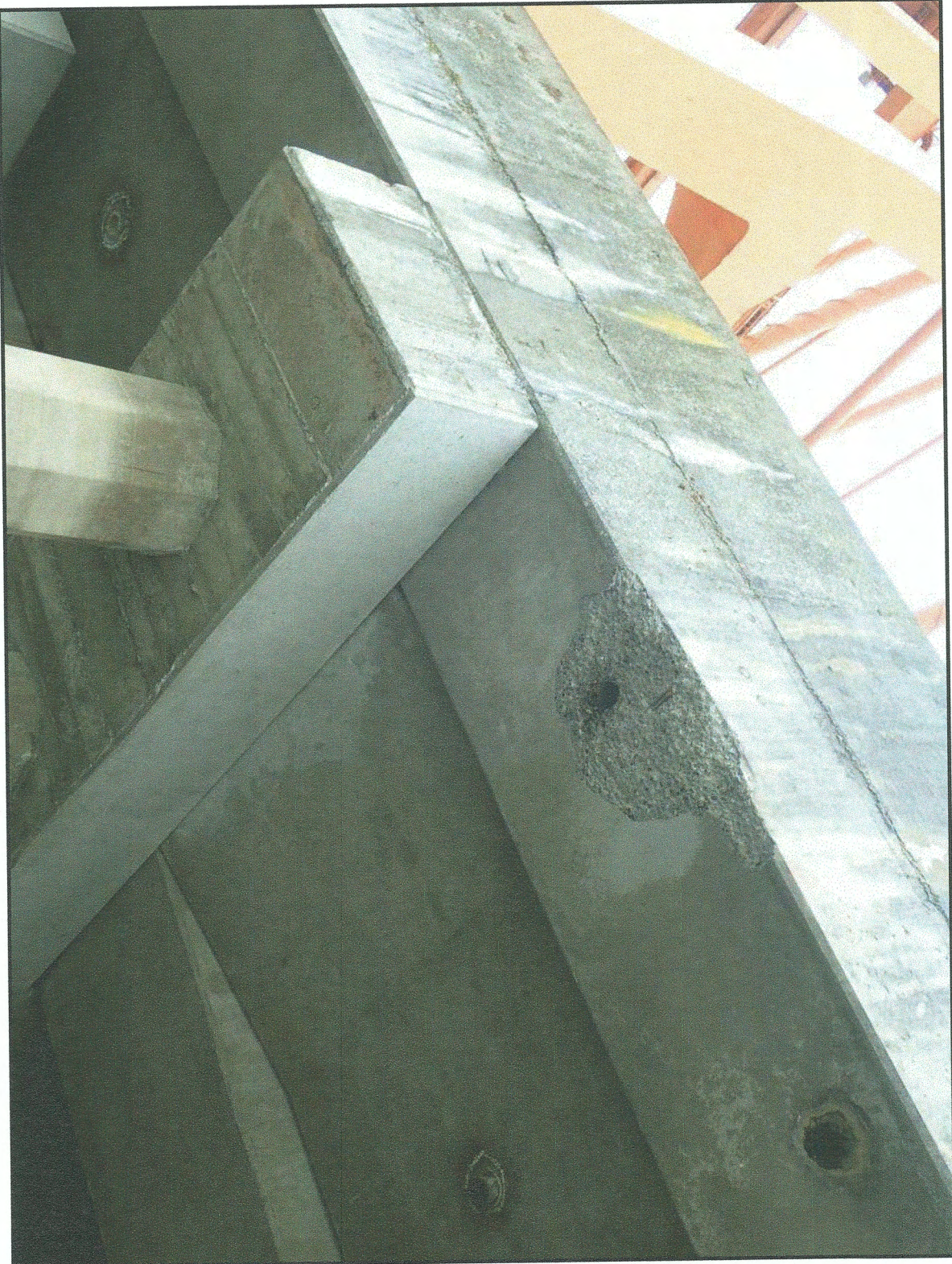
P1 - EDGE BEAM SPALL - BENT 19 LOOKING SOUTH
