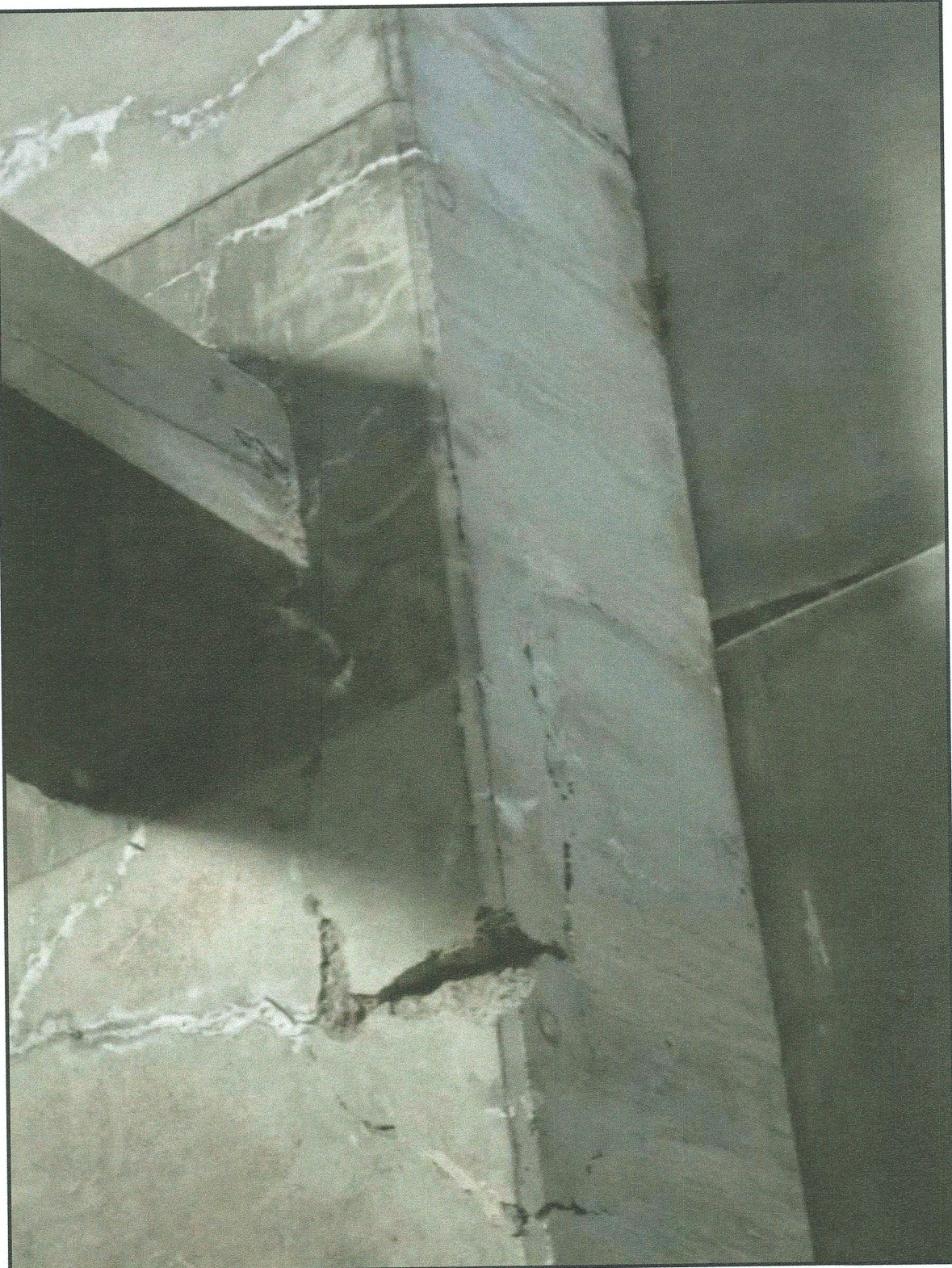
P2 - PILE CAP SPALL - BENT 82:B LOOKING SOUTH
