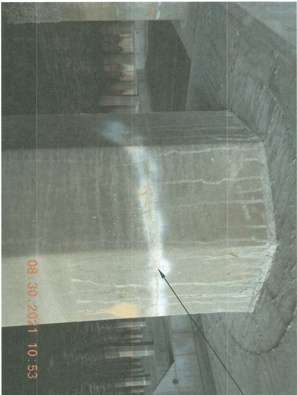
EXISTING CRACK, MARKED WITH WHITE PAINT
