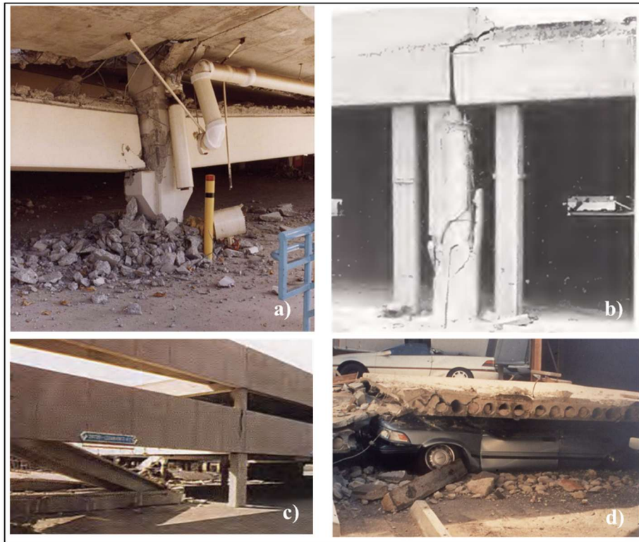
Figure 4 – Examples of poor design detailing that led to failure of precast gravity systems during the 1994 Northridge earthquake: a) failure of interior gravity column (fib, 2003); b) failure of exterior gravity column (Todd et al. 1994); c) unseating of double tee beam (Iverson and Hawkins, 1994); d) unseating of hollow core floor section (fib, 2003).
