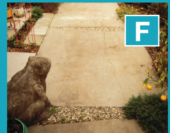
Horizontal 3"-6" cuts in walkway and driveway
