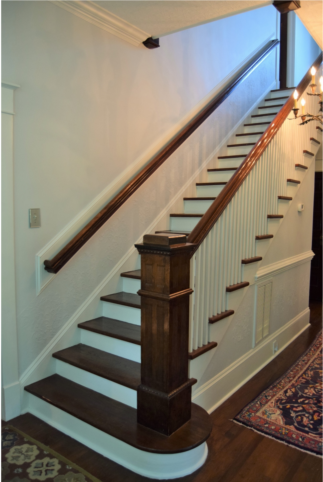
Roxana and Herman Greene House, Wake County, front stair, view to SW
