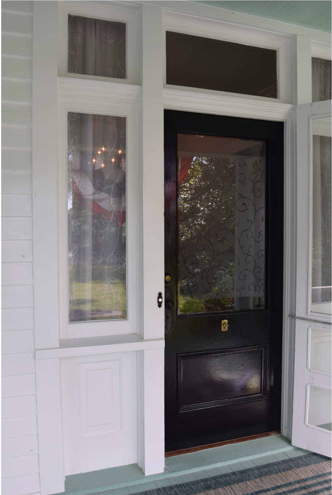
Roxana and Herman Greene House, Wake County, front entry, view to NW
